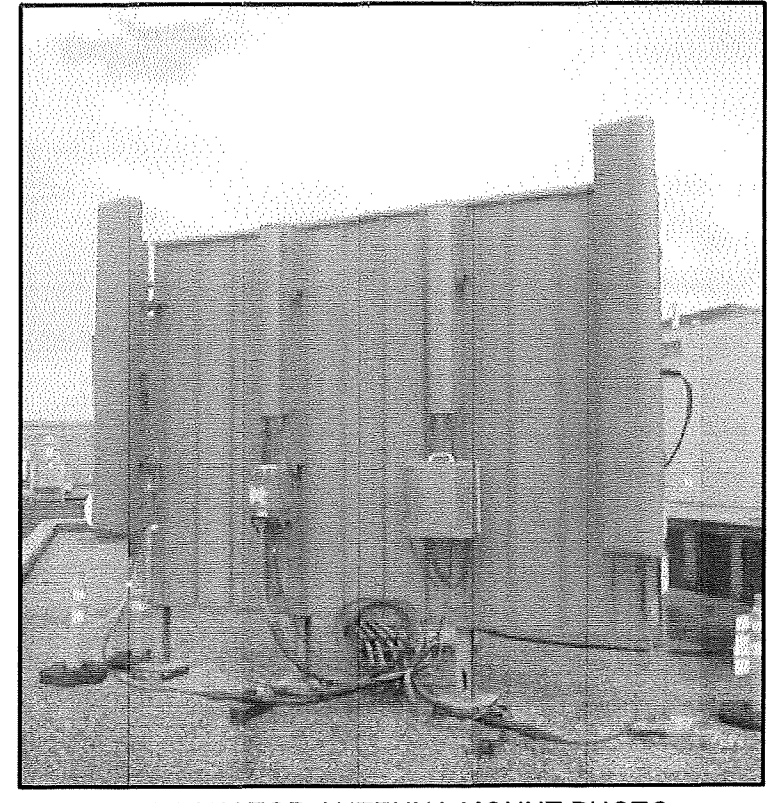
1 'Z' SECTOR ANTENNA MOUNT PHOTO SCALE: NONE
