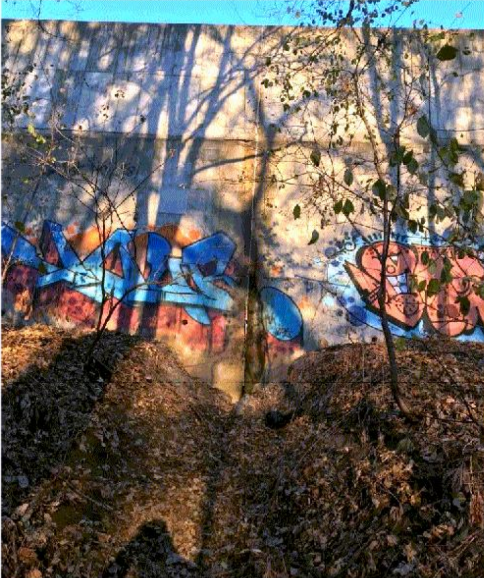
Figure 6. Drainage/Erosion Gully Located near the Center of the Retaining Wall on the Slope
