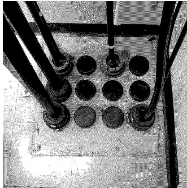
2 CABLE PORT PHOTO
