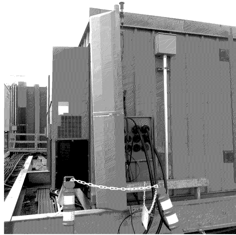
2 'Y' SECTOR ANTENNA
